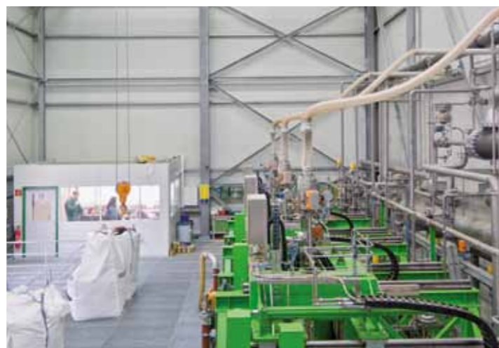
The heart of the system: the central control room (left) for the three extractors (right)
